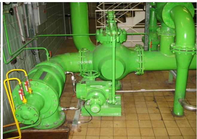
Figure 2. Pressure reducing valve in a cooling system [1]
