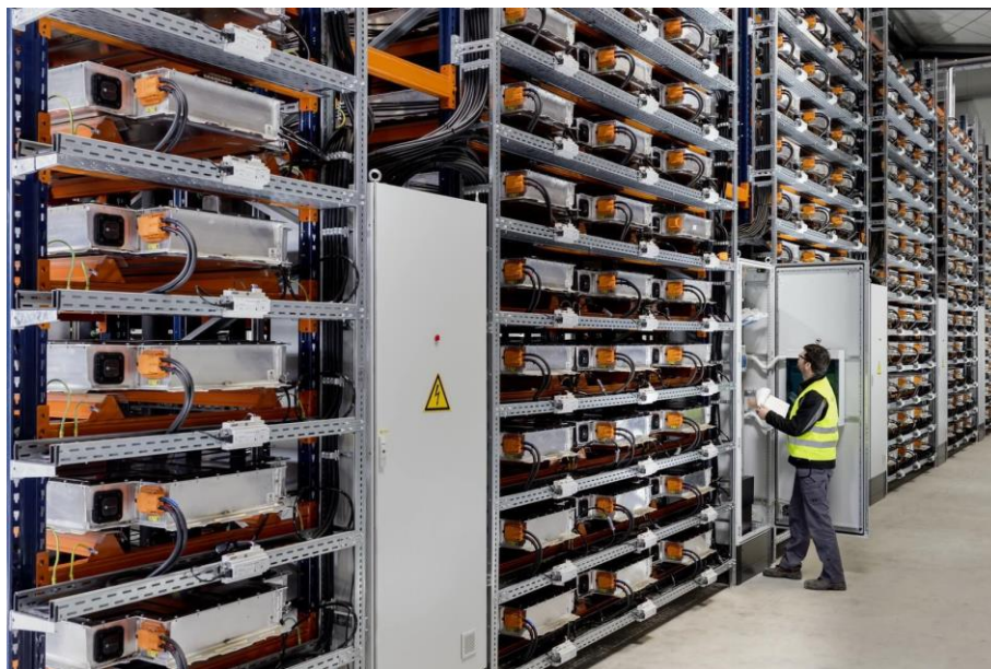
Figure 10: Storage of used BMW i3 batteries (BMW Group,2017)
