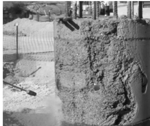
Figure 2. The upper part of the pile damaged by excessive bleeding
