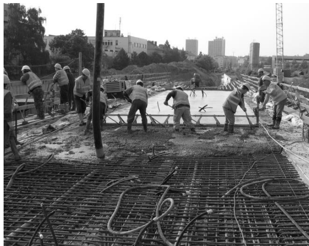
Fig. 2. Bridge deck construction, during which a sample of concrete B was taken to make test specimens.
