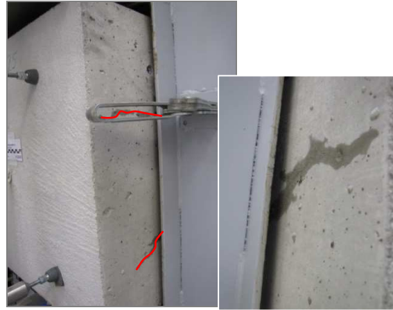
2. First cracks occurred on the all side walls generally in two-thirds (5 min)
