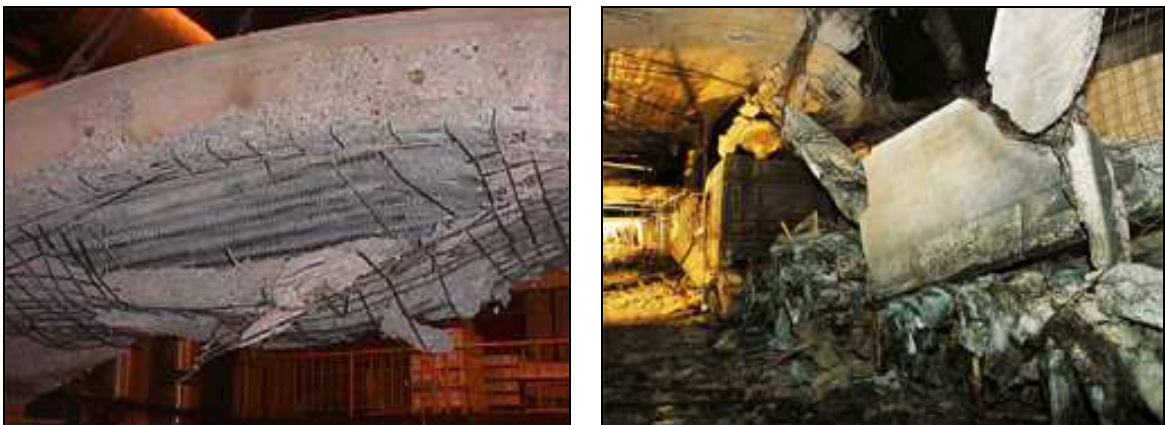
Figure 2-2: left: Uncovered reinforcement due to explosive spalling; right: Collapse of structure due to explosive spalling [17]
