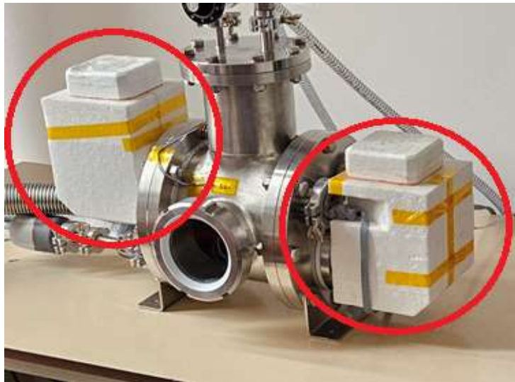
Figure 4.2 Isolation of LIN tanks
