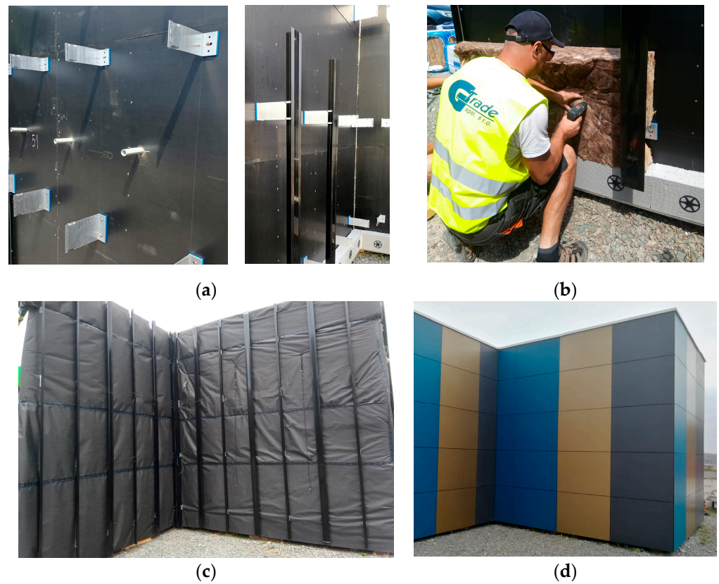
Figure 2. Construction of experimental block of façade: (a) base wall with a grid of aluminum brackets. The upper row of brackets is built from sliding wind load brackets, while the bottom row are fixed brackets that also carry the weight of façade; (b) installation of thermal insulation; (c) finishing the thermal insulation with a protective layer and a grid of supporting aluminum T-profiles connected to the brackets; (d) finished façade.
