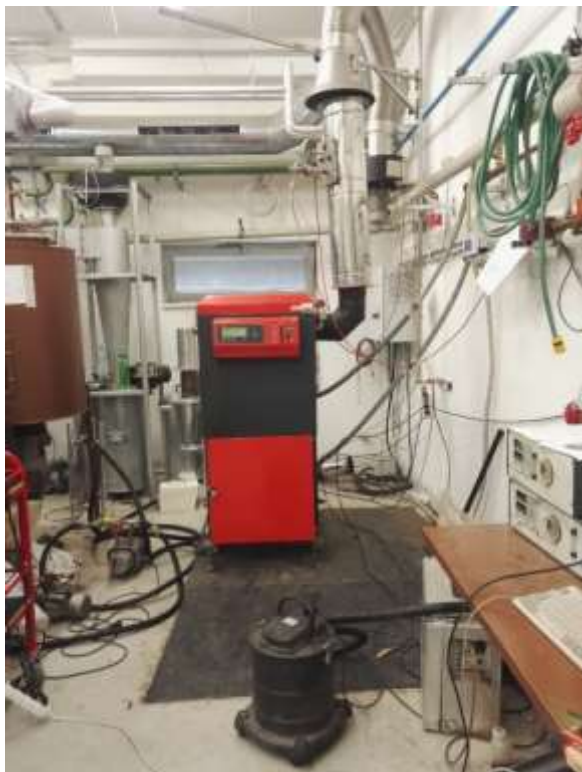
Obr.3.3 Kotel VERNER A251
