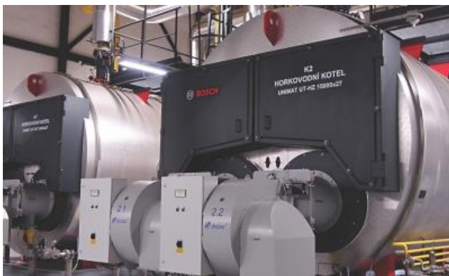
Obr. 1-3 Kotle v provozu Brno-Sever [23]
